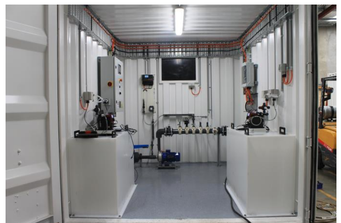
Custom SHDR plant with dual chemical dosing
