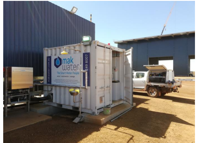
Containerised SHDR plant installed onsite
