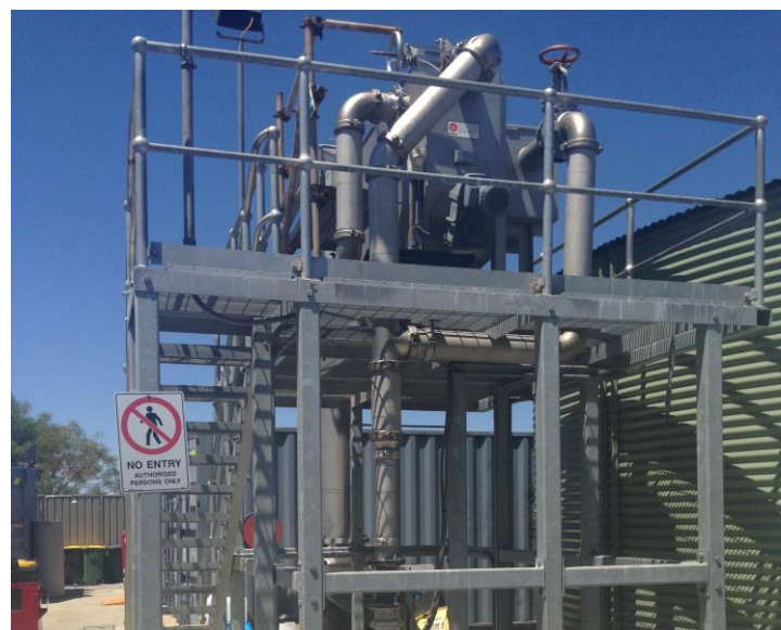
Pre-existing Sewage Treatment Plant (STP) MAK Water provided expertise and maintenance
