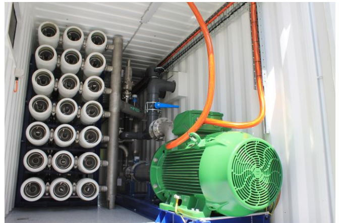
Containerised 1,272 m 3 /day Sea Water Reverse Osmosis (SWRO) plant
