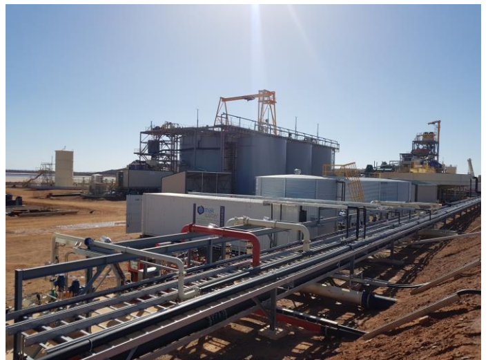
SWRO installed onsite at the Mill
