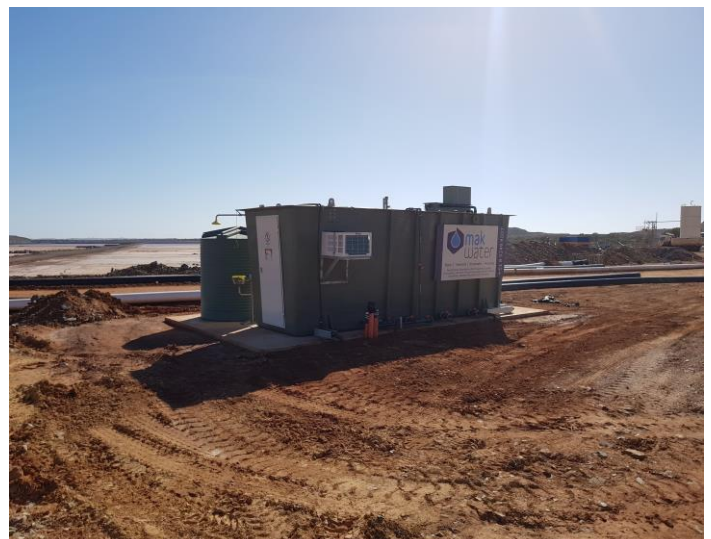
ASBR sewage treatment plant installed onsite
