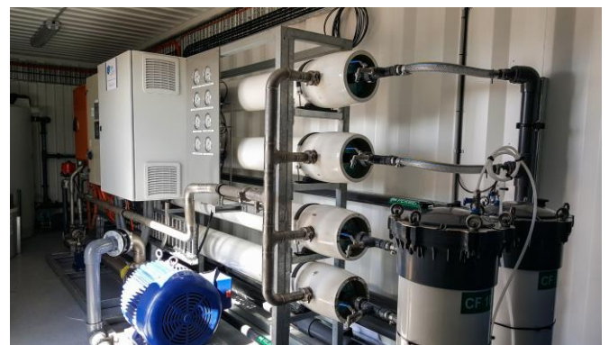
An inside look into a MAK Water SWRO hire plant
