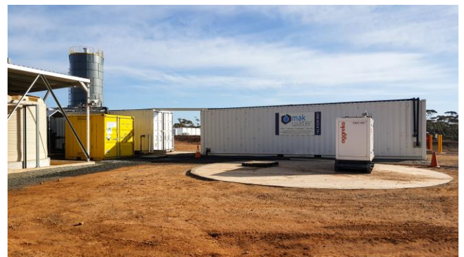
MAK Water SWRO hire plant installed onsite
