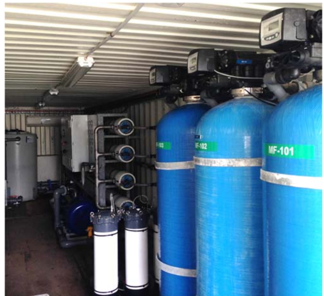
The Seawater Reverse Osmosis plant
