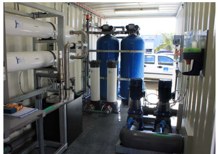
Containerised Sea Water Reverse Osmosis Plant with Chlorine Dosing and recirculation and monitoring systems.
