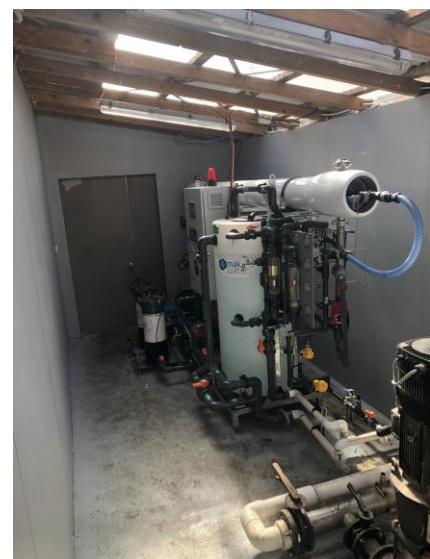
Custom Skid Mounted Sea Water Reverse Osmosis Plant - right view
