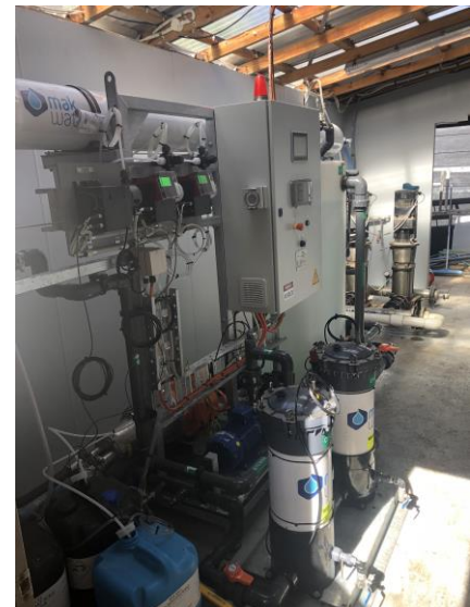
Custom Skid Mounted Sea Water Reverse Osmosis Plant - left view
