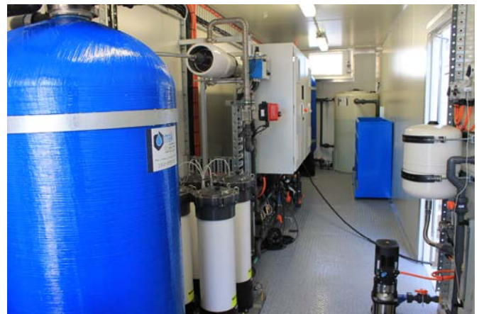
MAK Water containerised SWRO during factory acceptance testing
