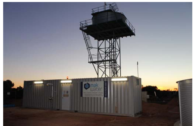
MAK Water containerised SWRO installed onsite
