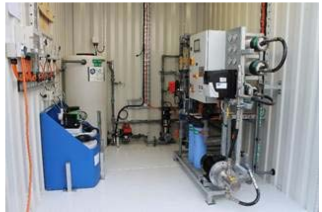
Sea Water Reverse Osmosis plant
