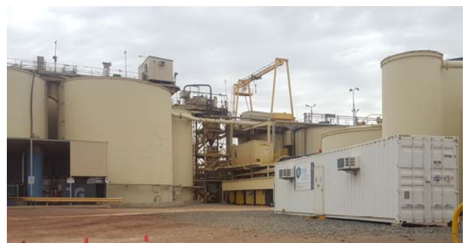
Sea Water Reverse Osmosis Plant on site in Laverton
