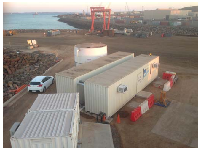
Sea Water Reverse Osmosis plant installed on site in Karratha
