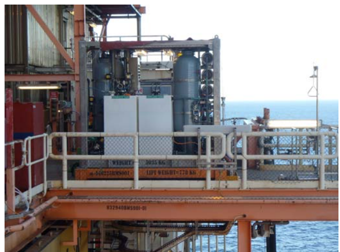
The sea water reverse osmosis plant installed on site on the offshore Goodwyn A oil platform
