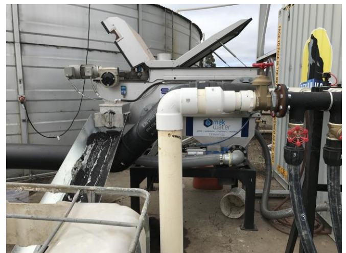
Salsnes Screen installed to reduce solids loading
