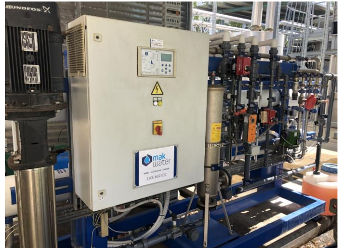
Probiotic Drinks Manufacturers' Reverse Osmosis Unit
