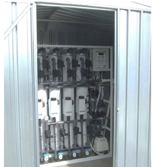
MAK Water UF-B package set up on-site in New Zealand
