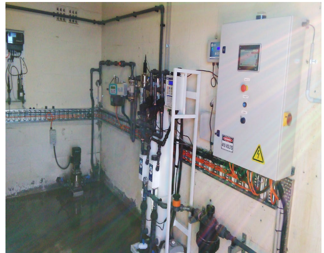
The installed 40 m 3 /day Siding Springs Observatory Drinking Water Plant
