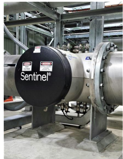
One of the two Calgon Carbon UV Technologies 24" Sentinel 9x10 UV reactors installed at Beenyup AWRP Stage 1
