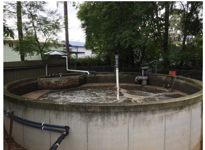
SBR Bioreactor with old 4kw aerator
