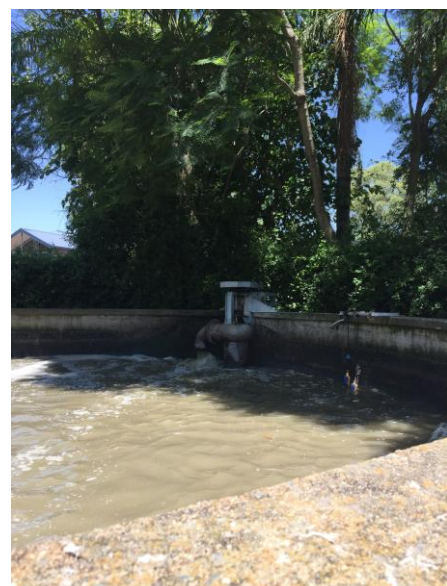
SBR Bioreactor with 7.5km submersible aerator installed
