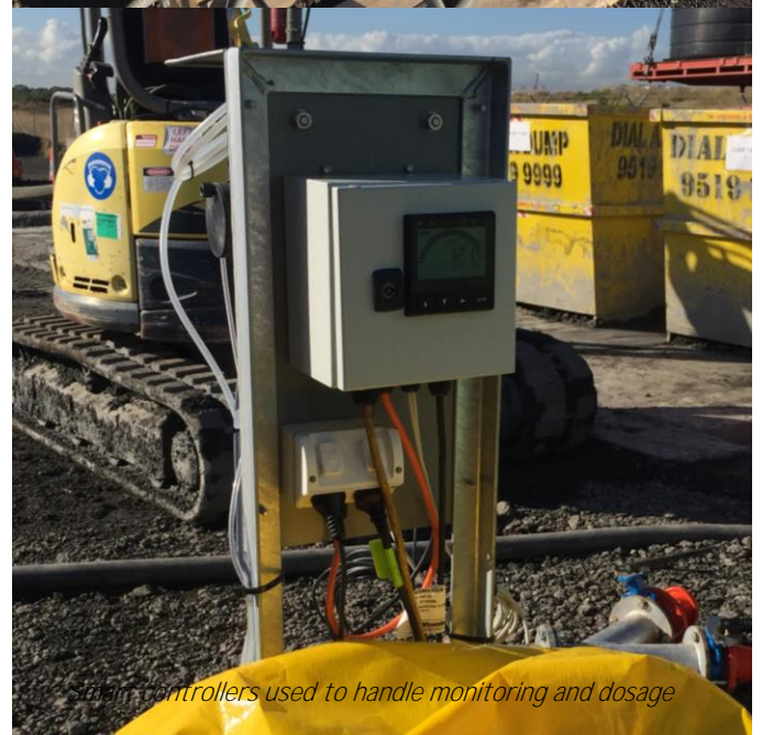
pH monitoring with automated control dosing unit
