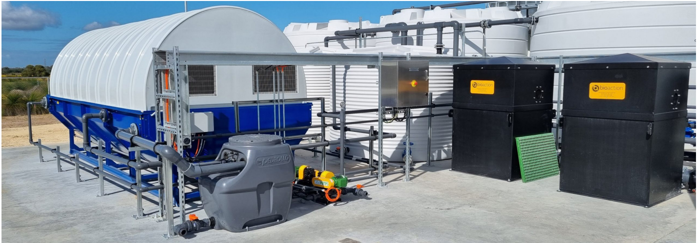
Biocombi Treatment Plant
