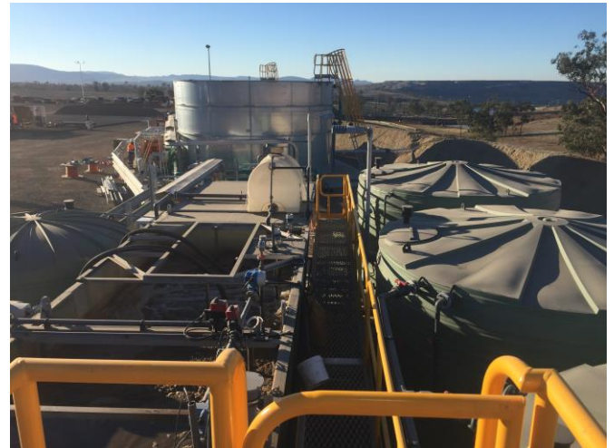
Membrane Bioreactor (MBR) Sewage Treatment Plant onsite in NSW
