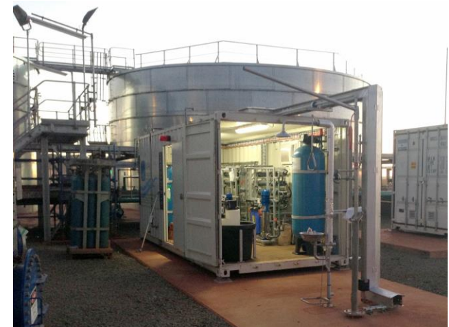
MAK Containerised 25 m 3 /day DWRO Plant
