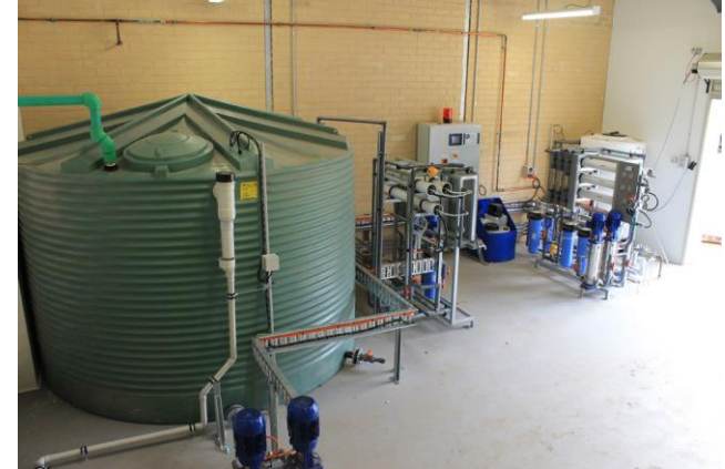
MAK Skid Mounted 10 m 3 /day DWRO Plant
