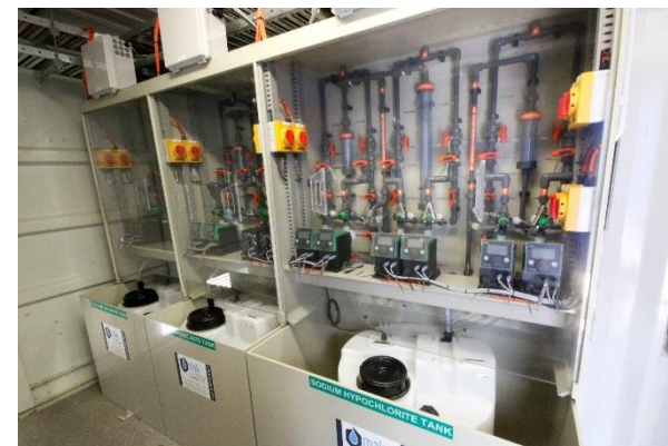
Acid, caustic and sodium hypochlorite dosing systems
