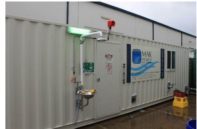
Containerised WTP with access door, window, safety shower & eyewash station
