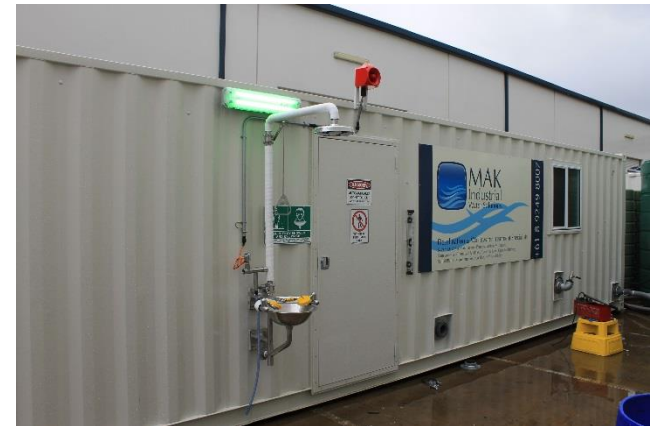
Containerised WTP with access door, window and safety shower & eyewash station
