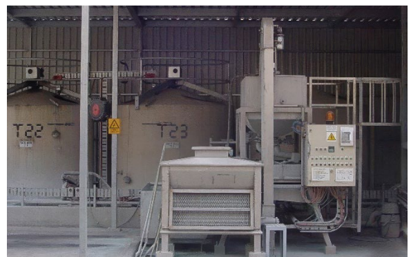
Single-Step Wastewater Treatment System (BCU) on site
