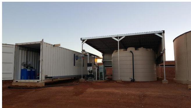
Containerised 240 m 3 /day BWRO plant installed onsite
