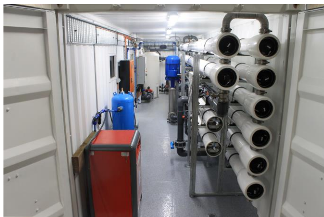
1,000 m 3 /day Brackish Water Reverse Osmosis Plant
