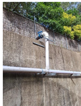
Water line entering the PHGC side
