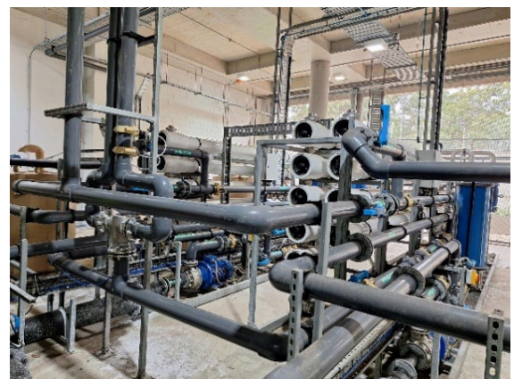
RO permeate flowing to NCX delivery lines
