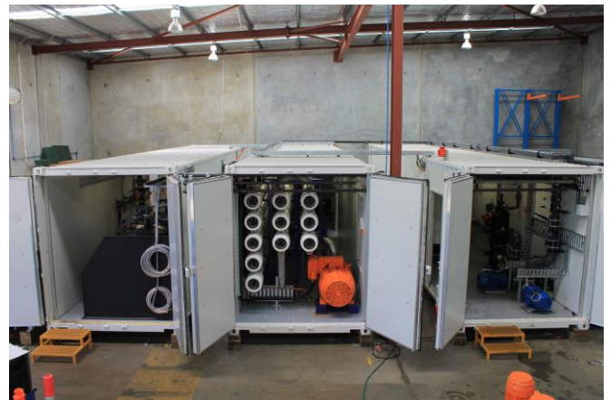
Containerised 1,310 m 3 /day high-recovery UF-SWRO plant undergoes factory acceptance testing
