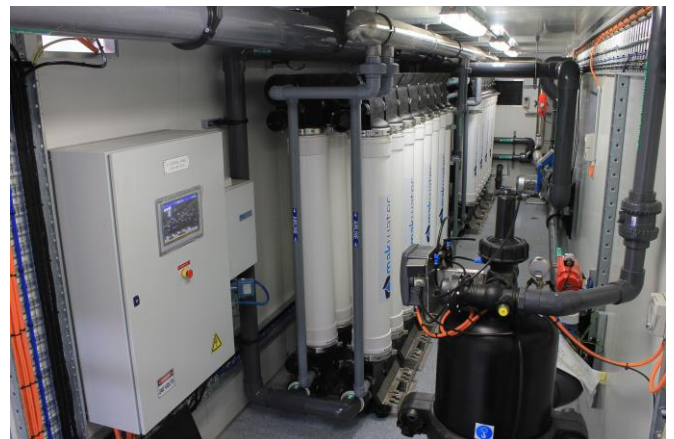
Robust cross-flow ultrafiltration (UF) pre-treatment was used due to high levels of suspended-solids in the feed water
