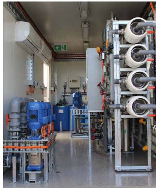
Containerised Brackish Water Reverse Osmosis Plant
