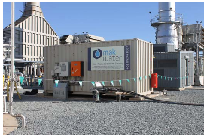
Brackish Water Reverse Osmosis Plant on site in South Hedland
