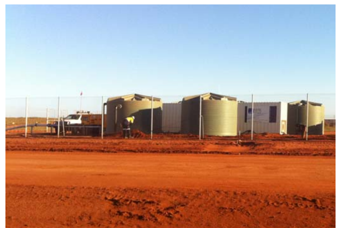
MAK Water provided all site installation works and commissioning as part of the turnkey solution provided to BHP Petroleum
