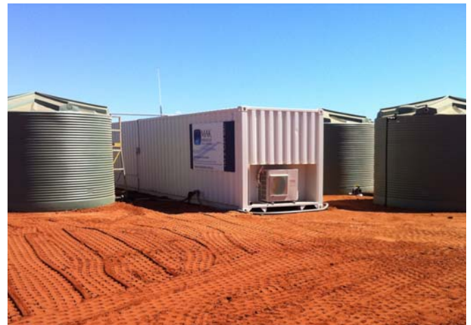
Brackish Water Reverse Osmosis plant on site
